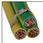
Stainless steel cable tie tensioned and cut i.e. no sharp edges
