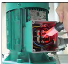
Incorrect phase sequence
